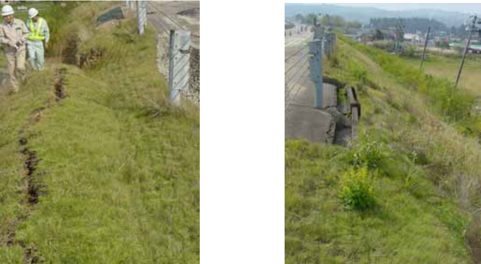
Longitudinal cracks at the top of the embankment (due to lateral movement)
