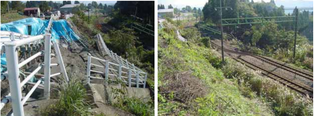
Slide-induced collapse of the railway embankment and road running above it
