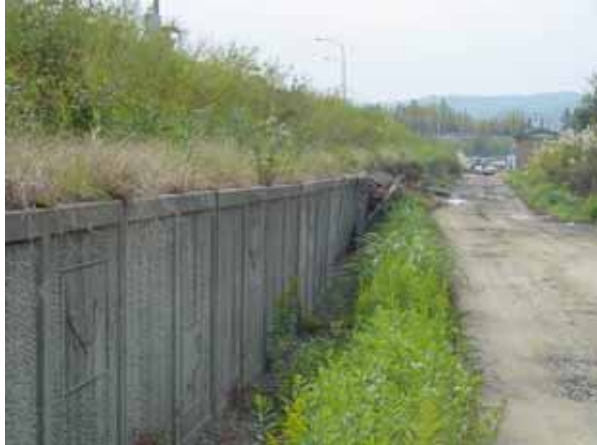
Lateral movement and collapse of the retaining wall (mountain side); Concrete culvert in the underpass of the highway
