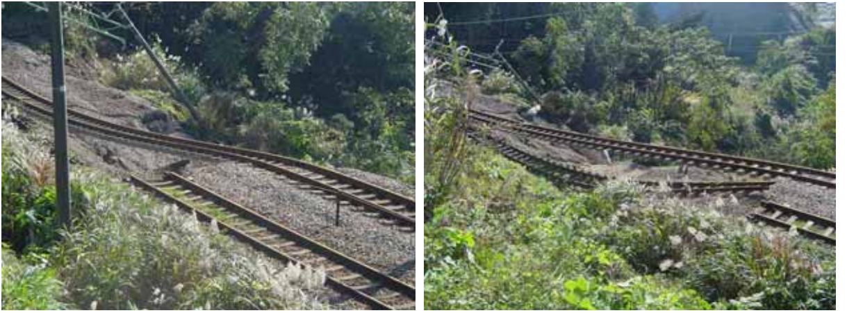
Hanging railways over the collapsed portion of the railway embankment
