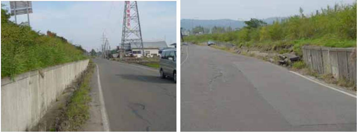
Lateral movement and collapse of the retaining wall at the foot of the embankment (Ojiya side)
