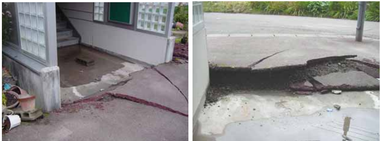
Differential settlement observed at the entrance of Bldg. 2
