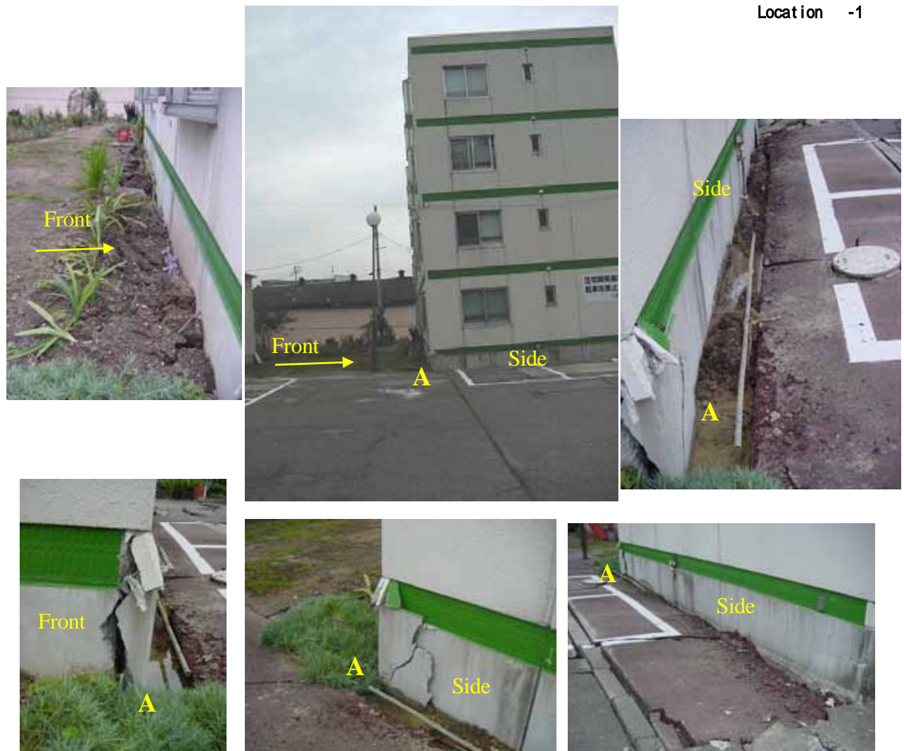
Bldg. 1 shown in the photos above tilted about 1°.
