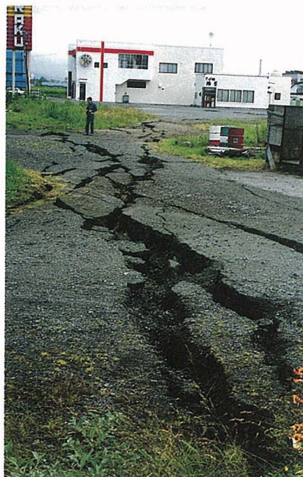
写真4-11 道路周辺地盤の亀裂 Ground cracks in the vicinity of the road
