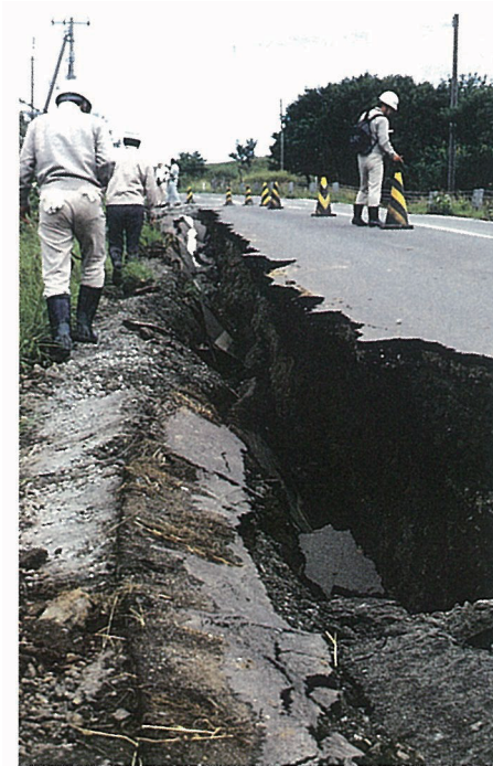
写真4-6 道路盛土路肩部の亀裂 Cracks on the side of the road embankment
