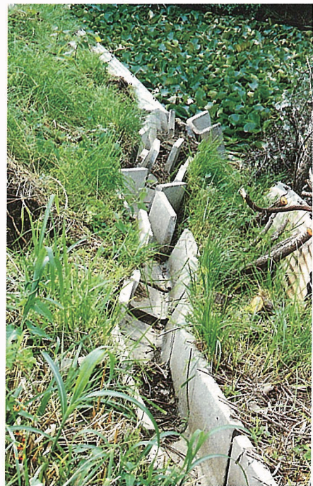
写真4-7 のり尻部のU字溝の変形 Deformed U-shaped channel on the side of the road
