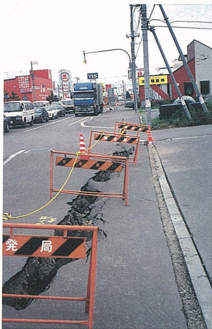
写真4-12 歩道の亀裂・陥没 Cracks and depression in the sidewalk
