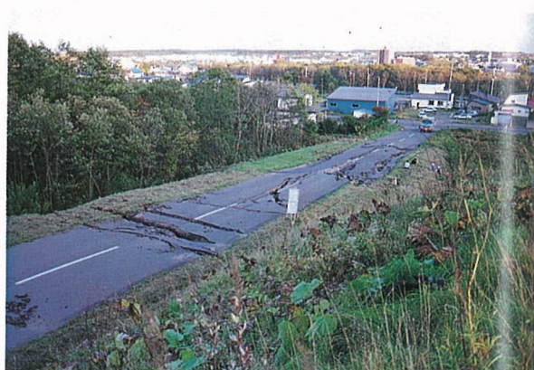
写真-5.8 隣接する道路の横断亀裂 Transverse cracks on the road which subsided
