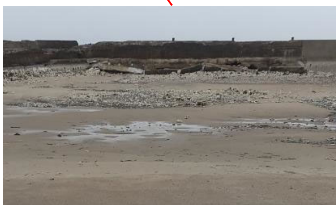
②防波堤の損壊
