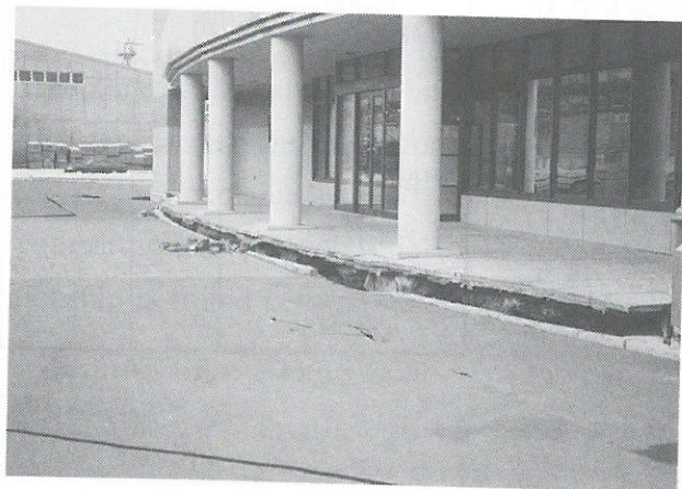
写真9.3 釧路港マリンプトスの被害 (Photo 9.3 Damage to the Building of Marine Potos, Kushiro Harbor)
