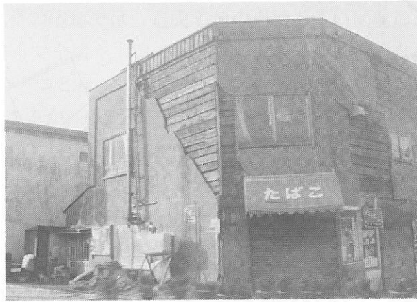
写真9.5 釧路市内のモルタル造の典型的な家屋被害 (Photo 9.5 Typical Damage to a Mortared House in Kushiro City)
