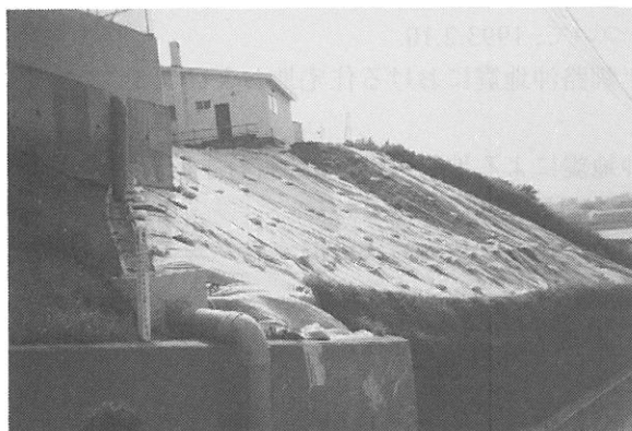
写真9.16 材木町の崩壊箇所の復旧状況 (Photo 9.16 State of Restoration of the Damaged Site in Zaimoku-cho)
