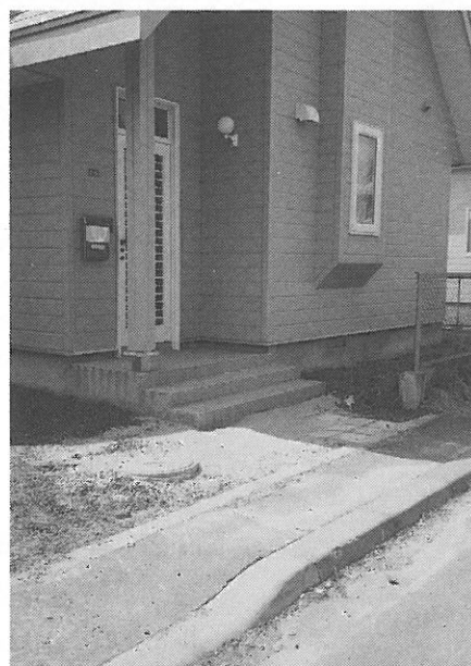
写真9.11 美原団地における噴砂発生状況 (Photo 9.11 Boiled Sand Observed at Mihara Housing Area)
