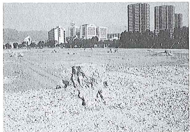
Fig. 9. Top of cast-in-place piles protruding above the ground surface
