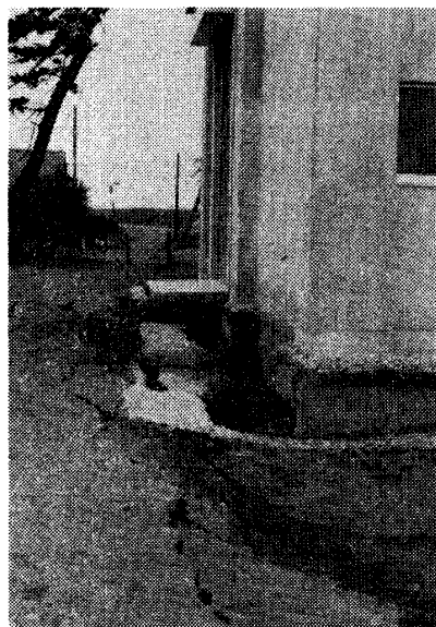
Photo. 18. An undamaged sewage plant (Arahama Gesuiro), and subsided surrounding ground (Site A-9)
