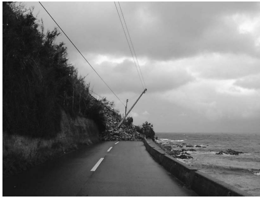
Photo 7 Slope failure in Shikano-shima island
