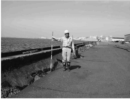
Photo 3 Displacement of a quay wall and subsidence of the ground in Oki-hama
