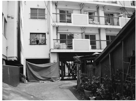
Photo 8 A damaged apartment above the Kego Fault
